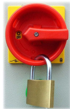
Fig. 58 Main switch secured
